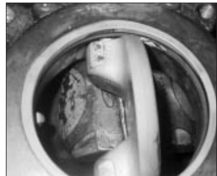
Figure 1 – shows the valve properly clamped in place
