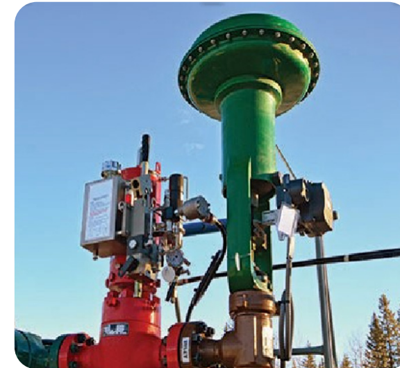
Pneumatic Automated Wellhead Choke Valve
