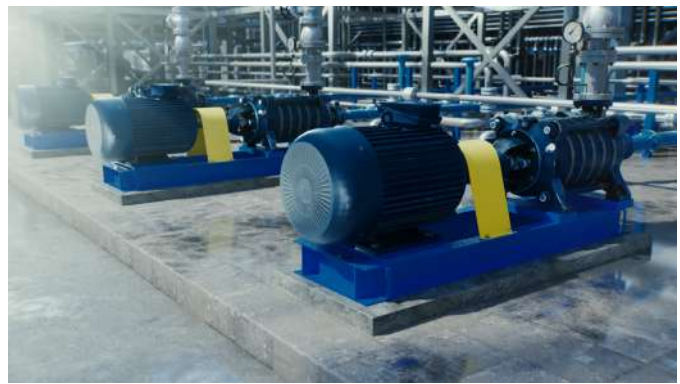
Figure 3-111: Surface Temperature Monitoring on Pumps.
