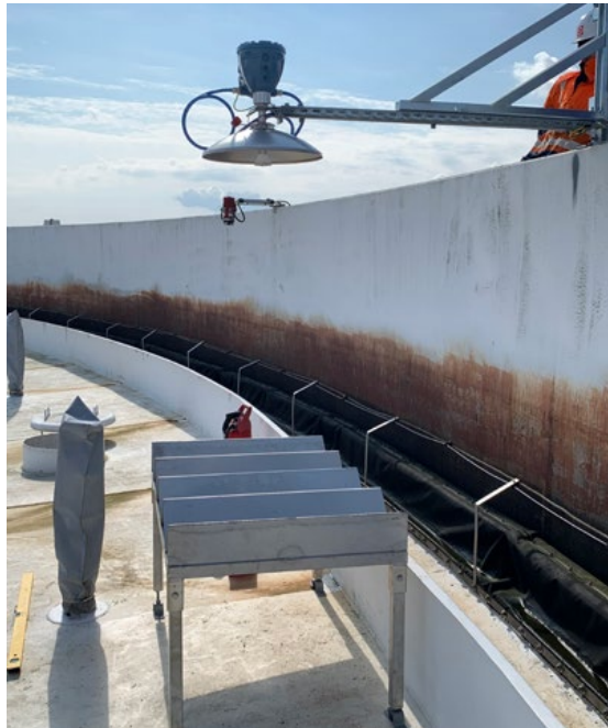
Floating roof monitoring with a target plate ensuring proper signal reflection from the radar level gauge.
