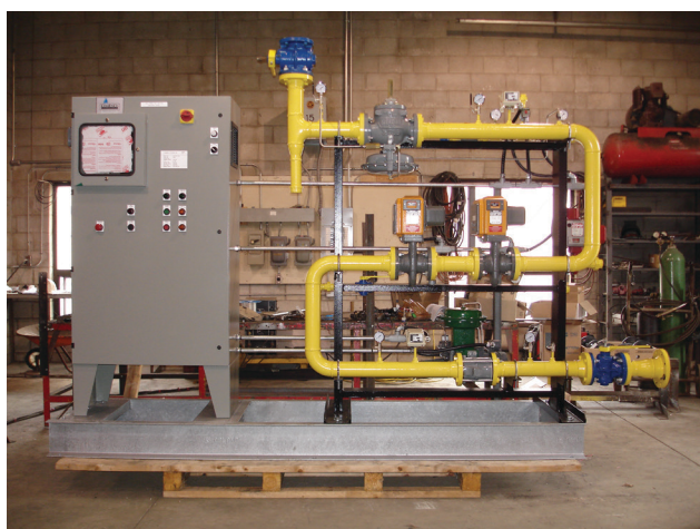
Figure 1. This turn-key fuel gas skid utilizes the highly accurate Fisher Type 1098-EGR pressure regulator to supply gas to a steam boiler.
