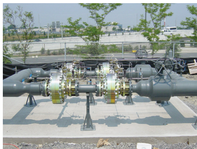
Figure 2. At the Toronto International Airport power plant Tartarini™ 6 in. Type FL pressure regulators are used to supply boiler fuel gas for steam generation.
