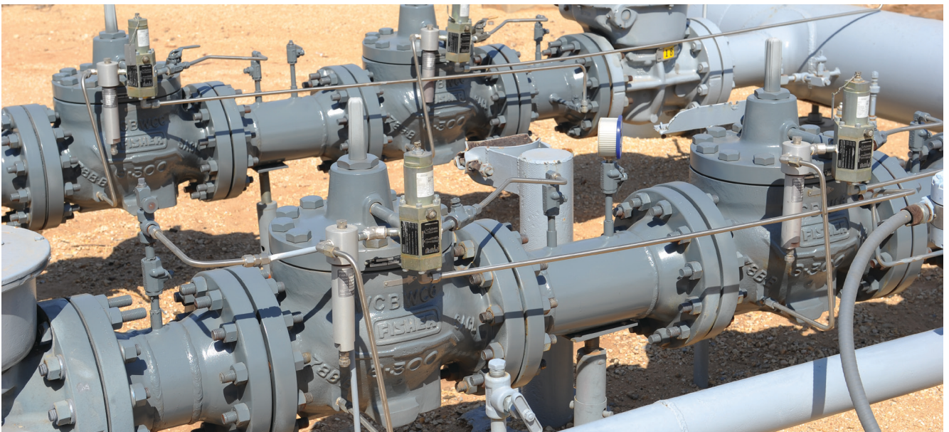
Figure 1. Natural Gas Distribution A typical dual run city gate station utilizes Type EZR's in a monitor configuration.
