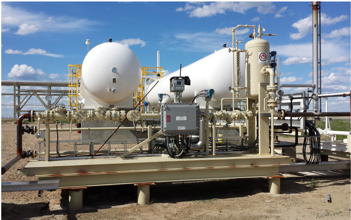
TruckVue™ NGL Transfer Point
